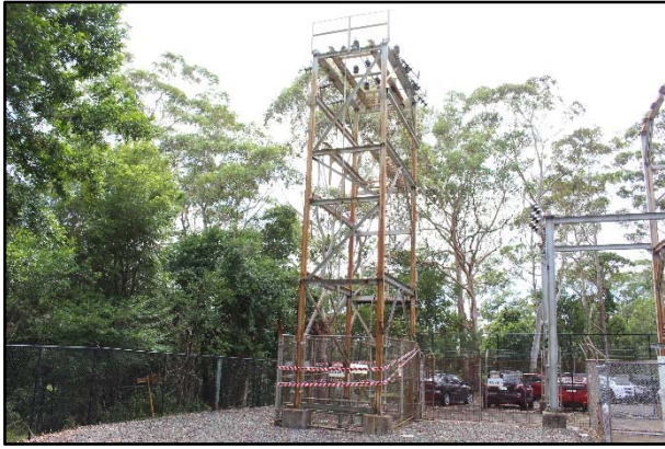
Plate 5: 3 m by 4 m steel tower to the north end of the compound, west aspect. (Source: Niche 2018).
