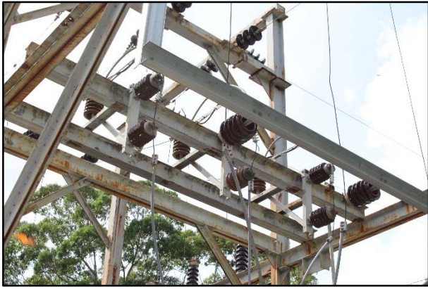
Plate 11: Example of orange brown ceramic transmission insulators, south east aspect (Source: Niche 2018)
