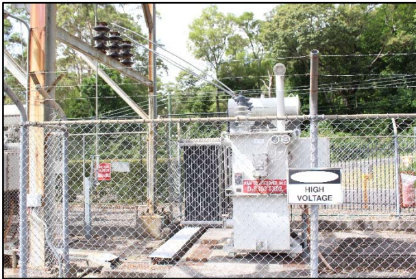
Plate 9: Example of modern transformer addition, south aspect. (Source: Niche 2018).
