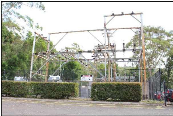
Plate 7: 4 m by 15 m steel tower to the south of the compound, south aspect. (Source: Niche 2018).
