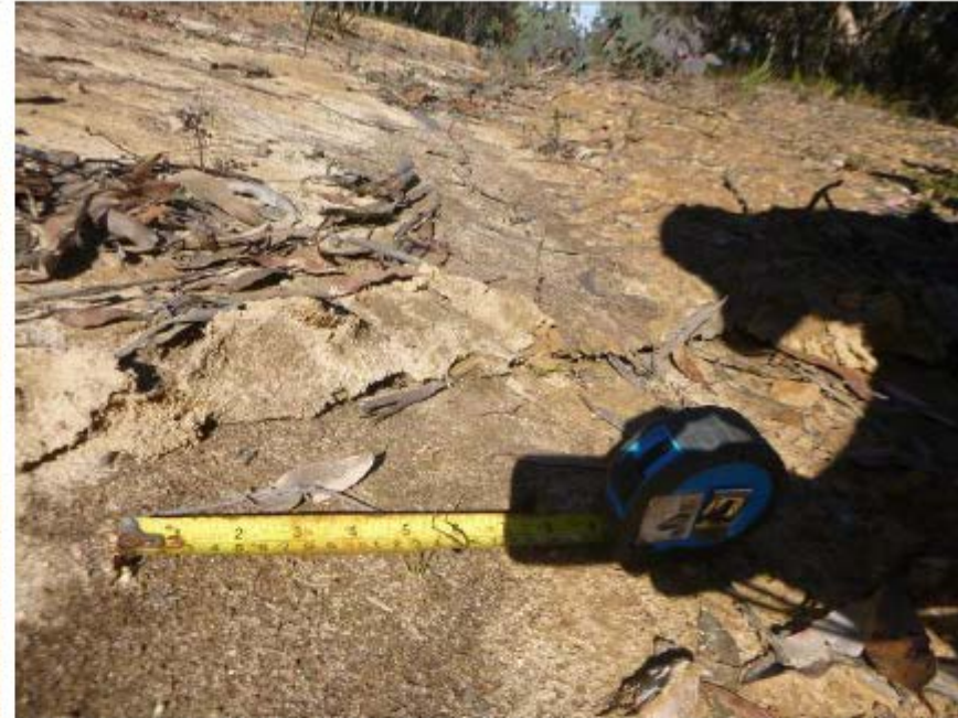
Photo 14: DA3B_LW11_001- Uplift on southern side of crack. Taken on 1/06/2015.
