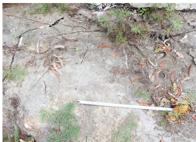
Plate 4: Subsidence cracking north of the shelter.
