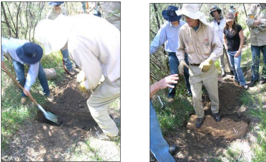
Figure 4-4 Trenching and Positioning of the First Layer of Coir Logs and Construction of a Small Dam in a Channel
