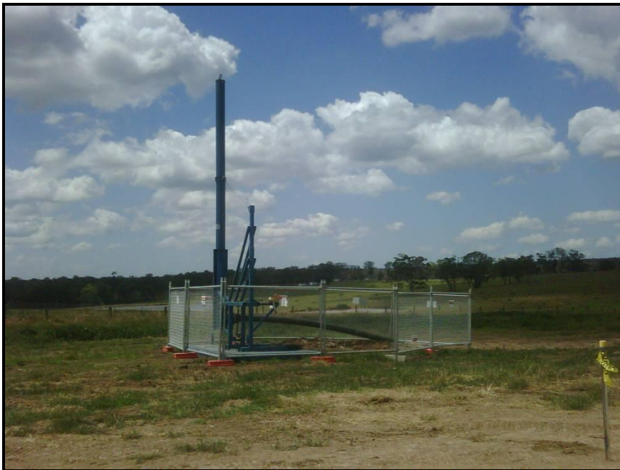
Figure 2.5 – Vertical Goaf Gas Discharge Stack
