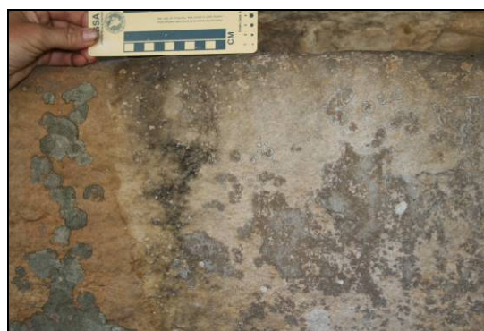
Plate 8: Example of water seepage and lichen growth on face of shelter
