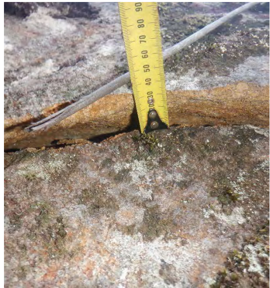
Photo 7: DA3C_LW21_026, Width of rock fracture. Taken 06/09/2023
