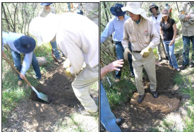
Figure 6-4 Trenching and Positioning of the First Layer of Coir Logs and Construction of a Small Dam in a Channel
