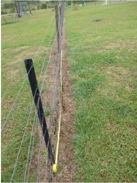
Photo 3: Cracking along fence line. Taken on 04/01/2016.
