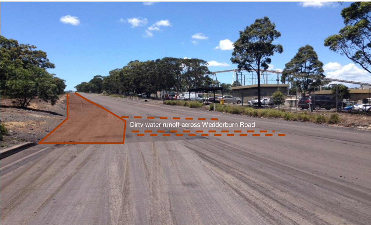
Figure 15: Drainage Issues at Northern end of Wedderburn Road (near Tarping Area)
