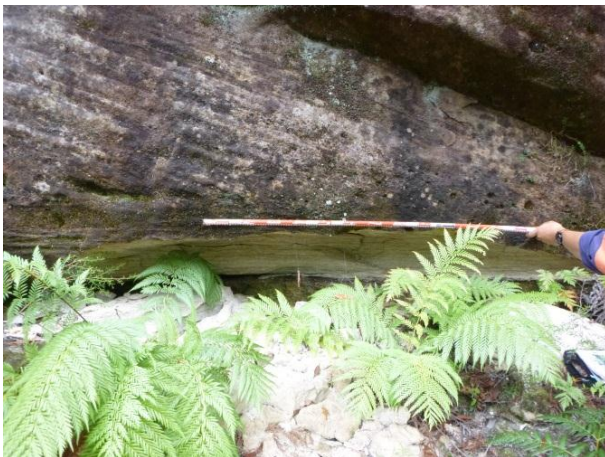
Photo 20: Impact DA3B_LW9_032 – Rockfall on outcropping. Taken on 06/02/2015
