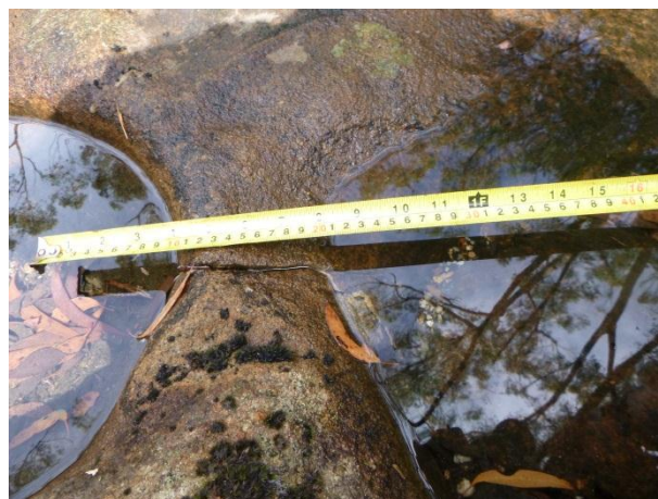
Photo 5: Impact DA3B_LW10_020 Fracturing to WC21_Rockbar 24. Taken on 02/02/2015
