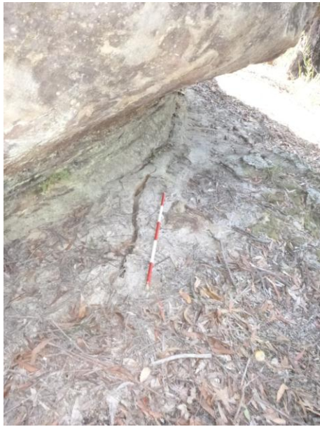
Photo 18: Impact DA3B_LW9_030 – Fracturing and soil cracking beneath step. Taken on 11/09/2014
