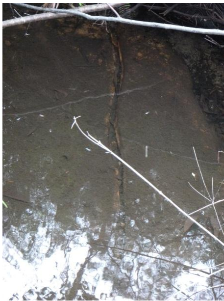
Photo 3: Impact DA3B_LW10_010 – Dilation of joint in base of pool. Taken on 25/11/2014
