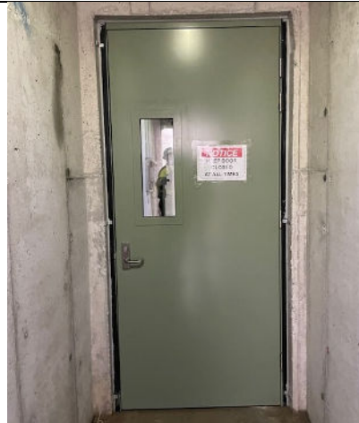
Plate 6: Acoustic doors in VS8 underground concrete encased ventilation system
