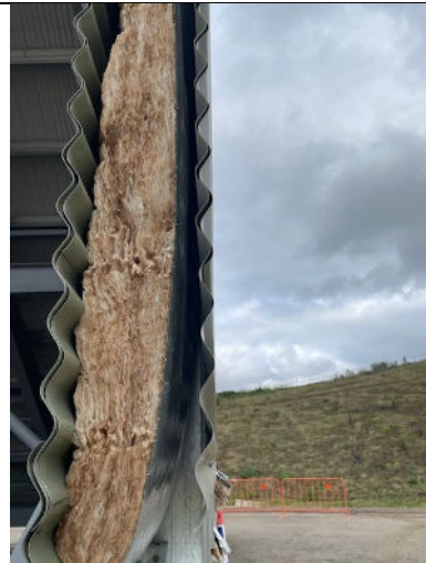
Plate 4: Double skin cladding and noise insulation
