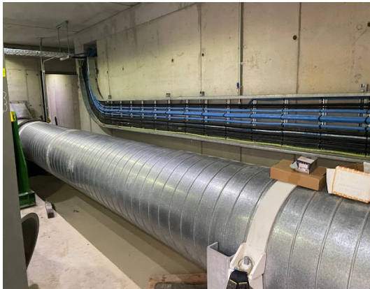
Plate 5: Underground concrete encased shaft ventilation system
