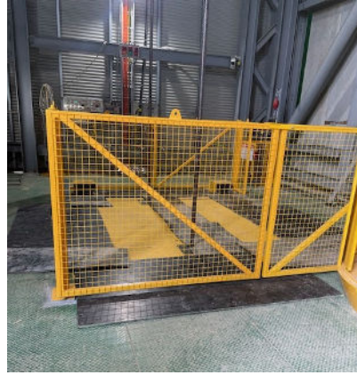
Plate 2: Heavy duty shaft blast doors
